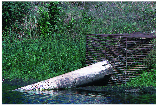
Figure 1: Perforated bottom intake pipe inserted into box-type parallel bar barrier at PDF 6 Pond. Some of the intake holes are exposed due to extremely low water levels during an extended drought.
