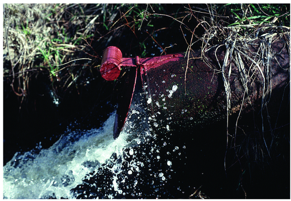
Figure 2: Flapper gate designed and installed by Foundation Wildlife and Fisheries Research Assistant John Holman on lower end of overflow pipe at PDF 6 Pond.
