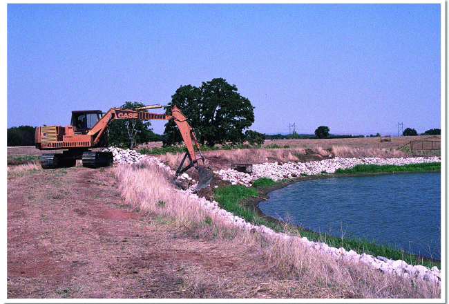
Figure 3: A riprap barrier being installed along the face of the dam at PDF 3 South Pond during drawdown to stop beaver excavation in the dam.
